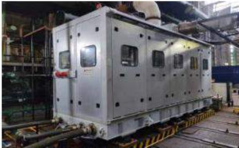
1000 KW Gen Set Installed in Acoustic Enclosure
